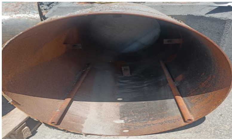
Figure 7. Coil damaged due to molten metal leak during sintering.
