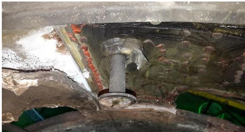
Figure 11. Burnt insulation layers on high temperature.
