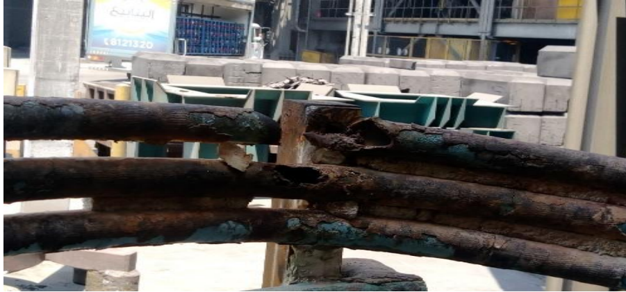
Figure 5. Coil damaged due to molten metal leak during sintering.
